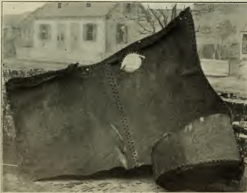
FIG. 2. SECTION OF SHELL OF THE EXPLODED TANK
